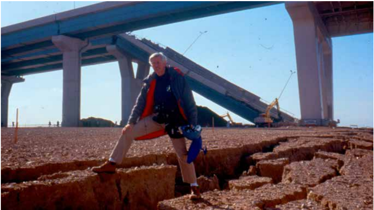
O'Rourke stands on ground deformed by liquefaction near the Nishinomiya-ko Bridge after the 1995 Kobe earthquake in Japan.
